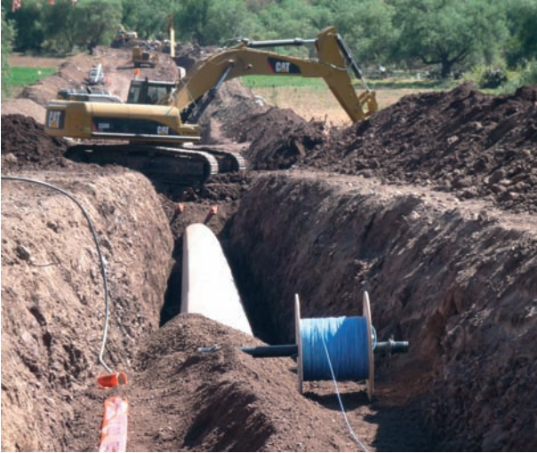
Example of sensing cable deployment during pipeline installation. On the left (orange) is the temperature monitoring cable, on the right (blue) is the strain monitoring cable.
