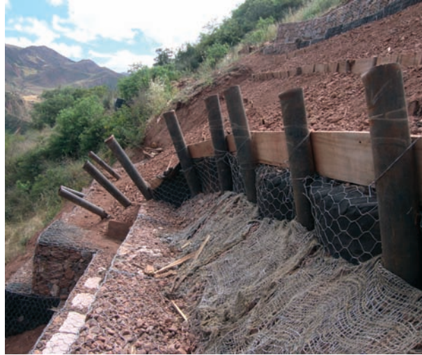
The right-of-way reinforcement is displaced by a landslide. Such events are detected and located remotely by DITEST-AIM.
